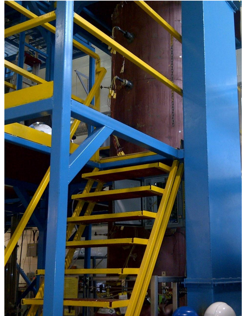
Storage tank (1.2 m x 5 m)
