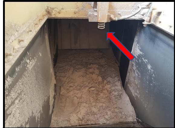
Inside of abort gate showing material build-up and activating spring assist
